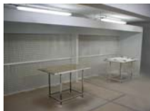
Caption: Hi-Tec Spray's "Twin Booth" system in-situ at Komfort Workspace PLC
